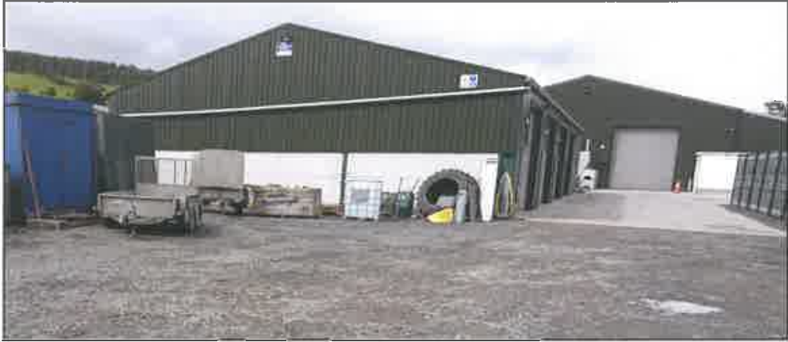
Figure 8: The existing shed south gable. Design and materials are to be the same
